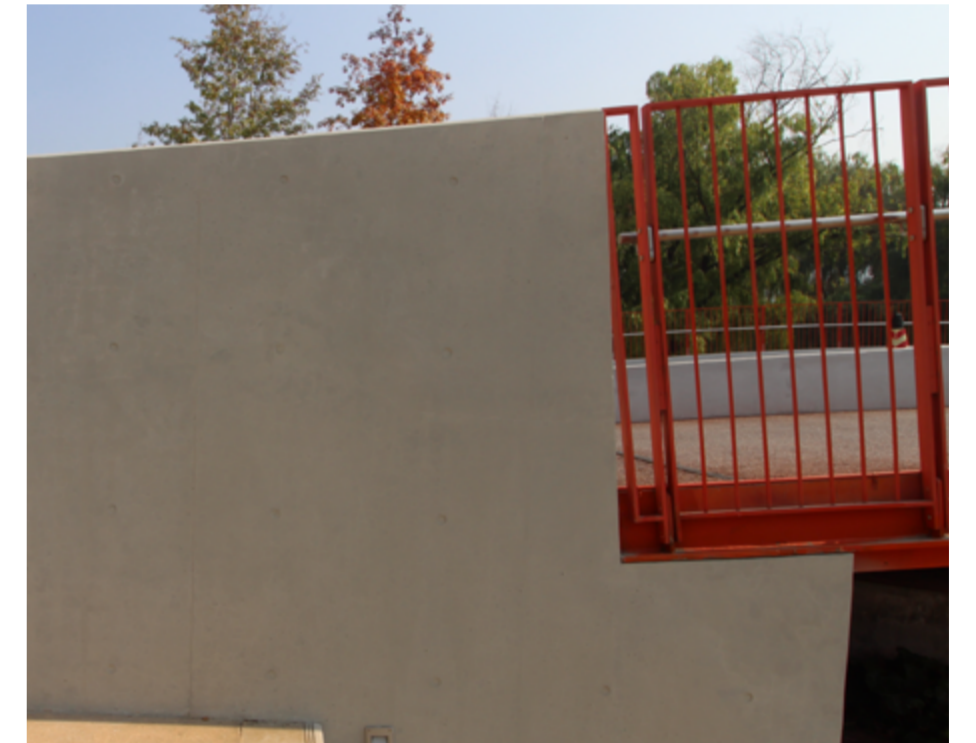
杭州天目里-红桥修复/OoEli-Red Bridge Repair Hangzhou - China Design by Renzo Piano Building Workshop
