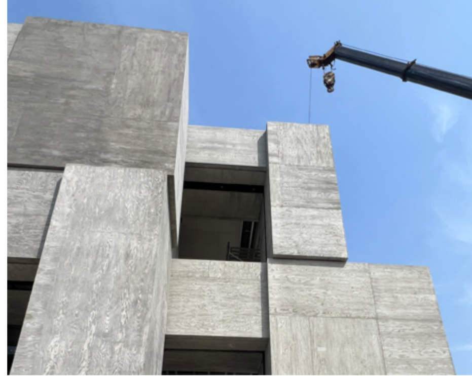
中国京杭大运河博物院二期/Grand Canal Museum Hangzhou - China Design by Herzog & de Meuron
